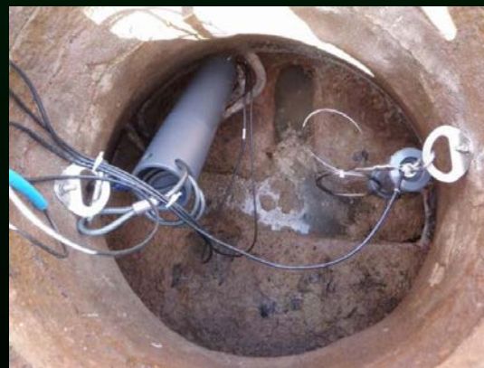
Flow/Water Level Monitors
