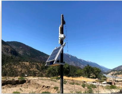
Mounted on pole, Point sampling
